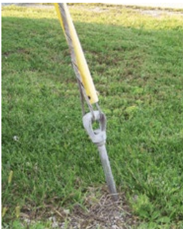
Utility Pole Anchor
