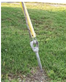
Ancrage de poteau de services publics
